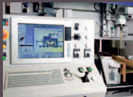
Mobile control panel
